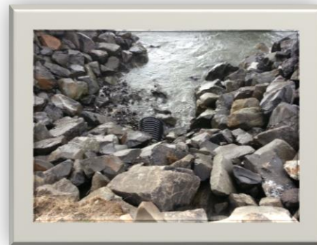
Figure 3.25 – Image of Outfall AD
